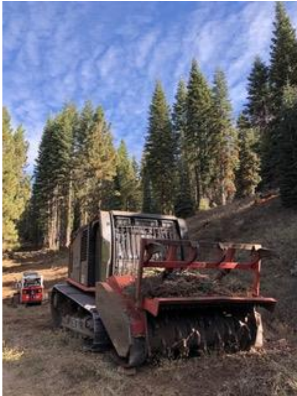
Masticators: These machines are called masticators and they remove small trees and vegetation using drums with teeth spinning at high speeds.
